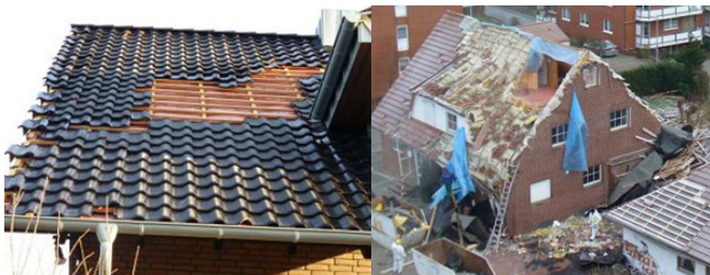
Roof tile damage is commonly observed in residential and small commercial structures (left) while severe roof damage (right) occurs less frequently (Source: AIR)
