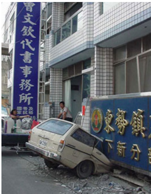
Figure 4. Soft Story Collapse in Chi-Chi (Source: AIR)
