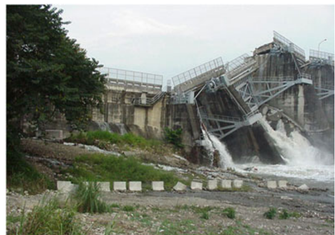
Figure 3. Partial Collapse of Shih-kang Dam (Source: AIR)
