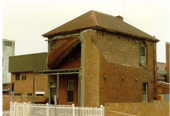
Figure 1. A double brick masonry wall damaged by the Newcastle earthquake (Source: City of Newcastle)
