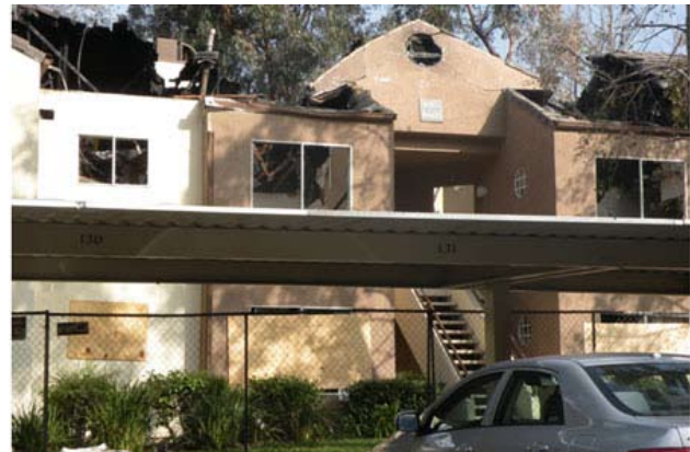
Figure 12. Numerous units destroyed at the Cascade Apartments. Source: AIR
