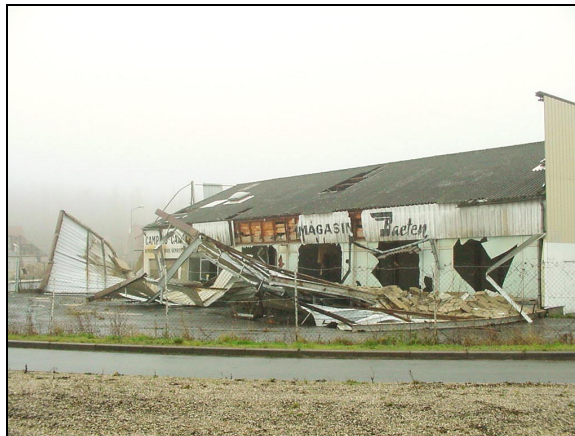
Damage to a light steel warehouse from windstorm Lothar.
